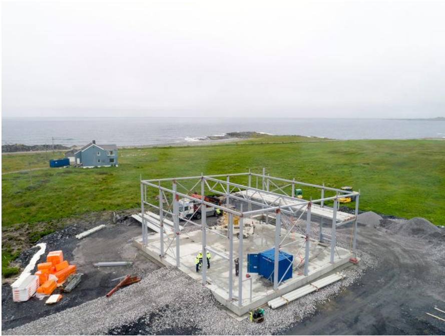
The building for the electrolyzer being constructed close to the port of the town of Berlevag. Photographer: Rocco Rorandelli for Bloomberg Businessweek
